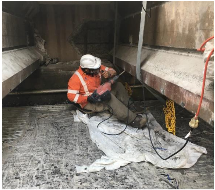
Figure 3b: Working underneath the structure and on top of scaffolding and capture sheet.
