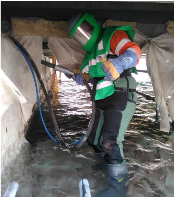
Figure 3a: Working underneath the structure and on top of scaffolding and capture sheet.
