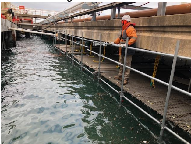
Figure 4: Temporary installation of scaffolding with a geofabric cloth used to capture waste from blasting infrastructure over water
