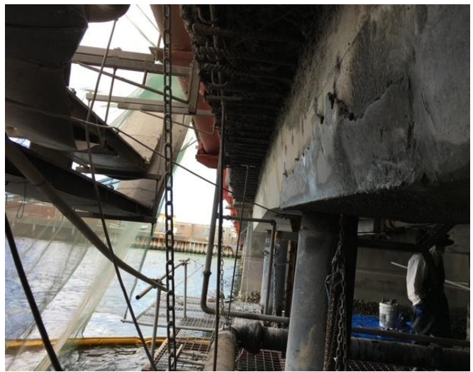
Figure 3: Temporary installation of scaffolding with a geofabric cloth used to capture waste from blasting infrastructure over water
